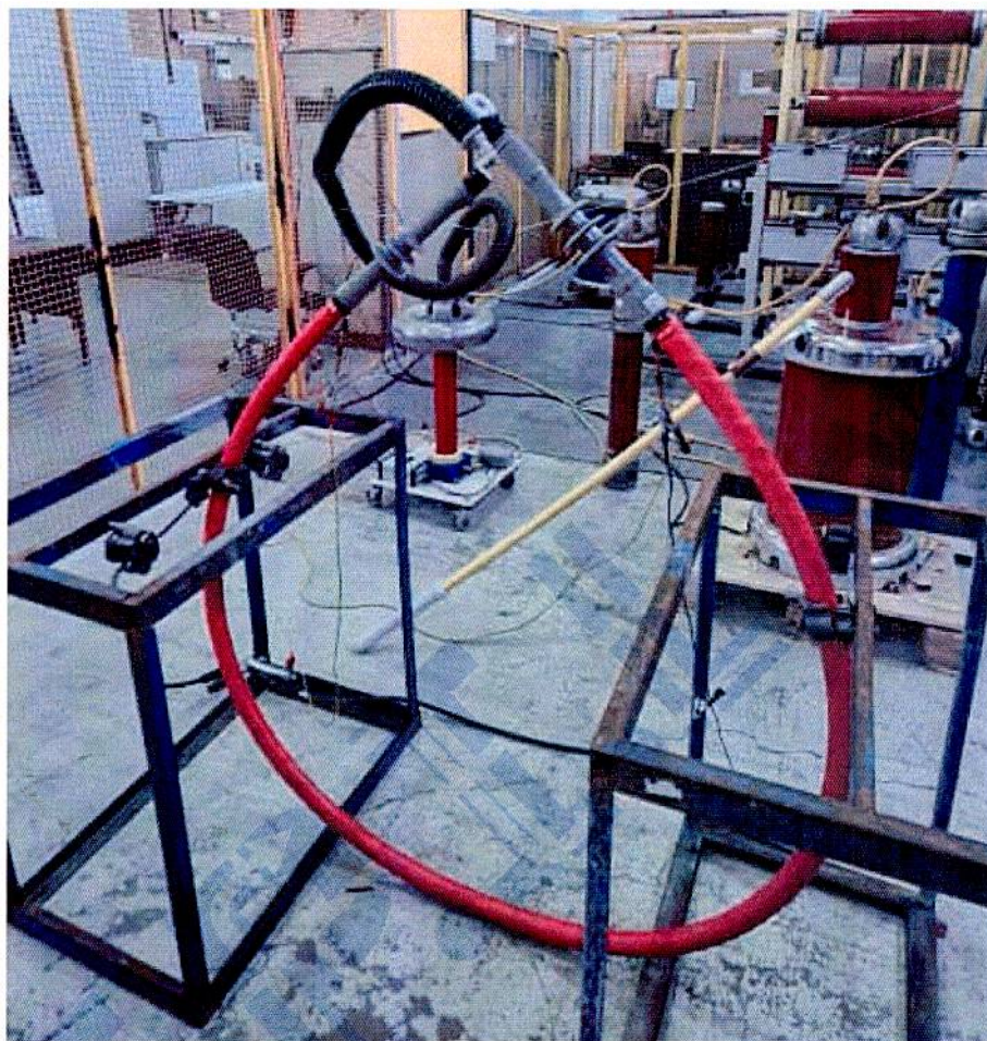
Figure 2. Equipment under partial discharge test
